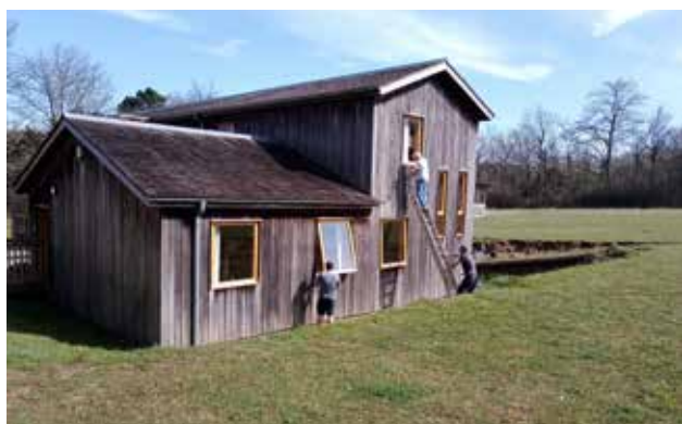
Window and door renovation project at Groundwork South Goblin Combe Outdoor Learning Centre in Cleve, supported by Community Fund grant.
